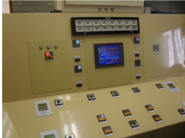
Pump Control Center
